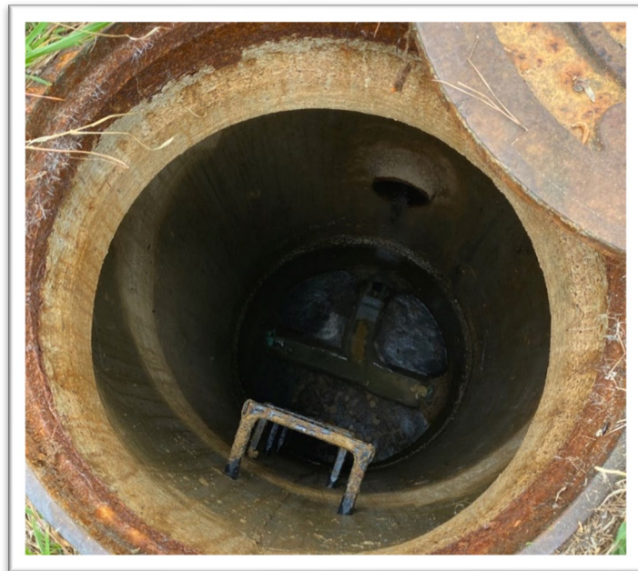
MH FID 43, BRINKLEY DRIVE, POOR.
