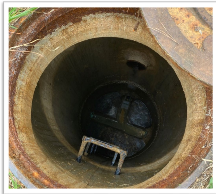
MH FID 43, BRINKLEY DRIVE, POOR.
