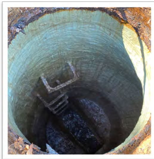
SMH 028044, Main Street in Wade. Rehabilitated manhole with lining, some corrosion on frame.
