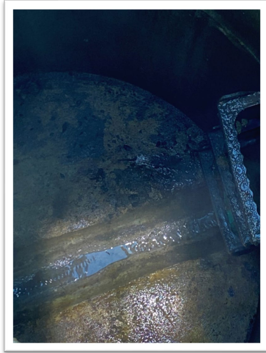
SMH-027203, Treadway Court. Precast manhole shows signs of corrosion and wear over time. Invert is well-formed.
